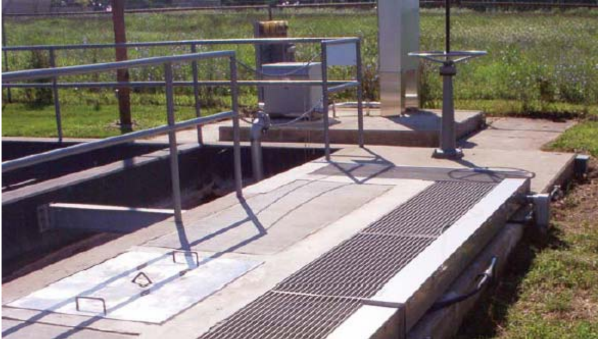
Figure 5-3: Low Pressure UV Disinfection System
