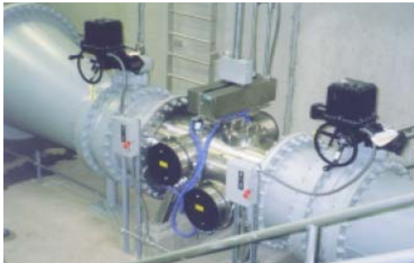
Figure 5-4: Medium Pressure UV Disinfection System
