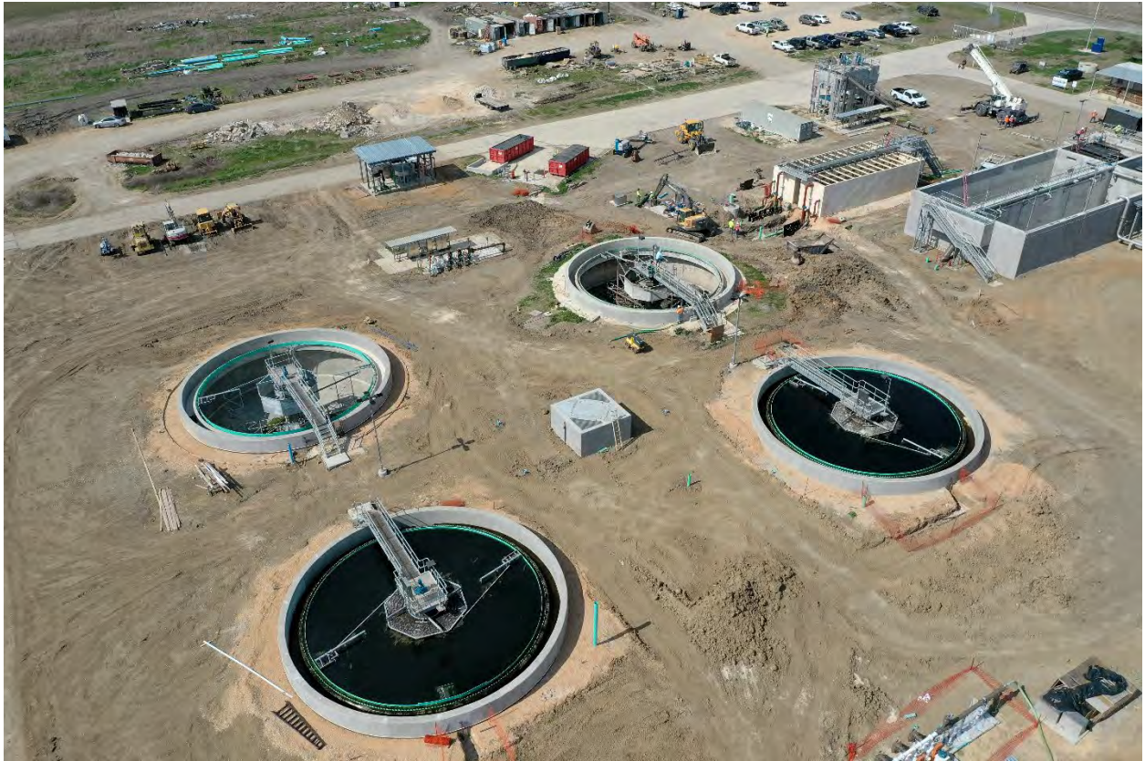
Martinez IV Wastewater Treatment Plant
